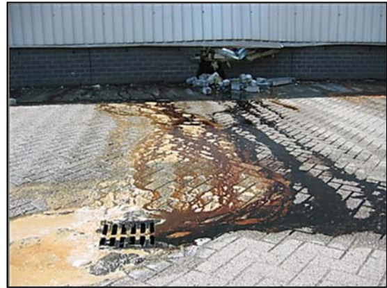
Image 12: racks against wall causing loss of containment outside storage compartment
